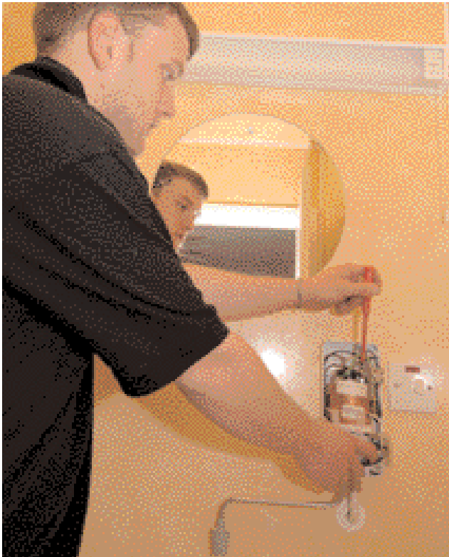
Electrical work in Bathrooms. High risk of electrocution if not installed correctly
